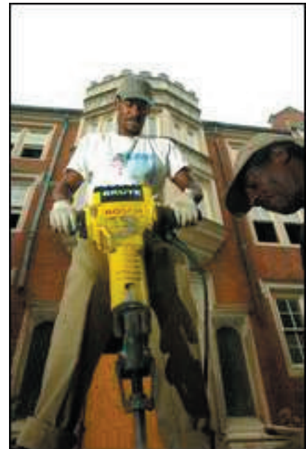
Breaking up concrete along the front foundation to make way for the new cooling system were Joelrico A. Payne, with jackhammer, and Timothy Byrd. Work began more than a year ago. (Photos by Keith Williams, The Courier-Journal)
